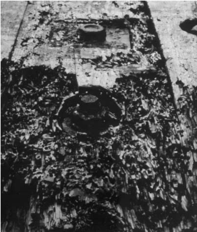
Fig. 5 Shipworm tubes in a lower plank of a floating fender from a watergate (Nordschleuse) in Bremerhaven harbours in 1998
